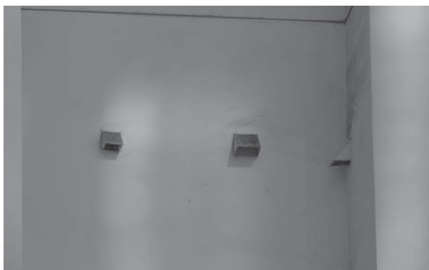
FIGURE 21.8 Exhaust ports on building facade. Note that the exhaust ports shown in this photograph are different sizes, corresponding to the different duct sizes. To create uniformity, the architect could require that all ports are identical in size. This would entail upsizing the smaller exhaust ports to match the larger ones. The ductwork size would not need to be increased; only the exposed shroud.
