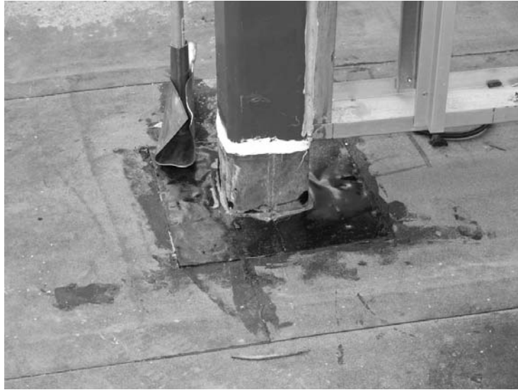
FIGURE 20.2 Lead roof jack. (Photo by author, courtesy of Hathaway Dinwiddie Construction Company and California State University Northridge.)
