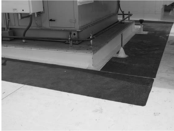
FIGURE 20.4 Walking pads. (Photo by author, courtesy of Hathaway Dinwiddie Construction Company and The California Institute of Technology.)
